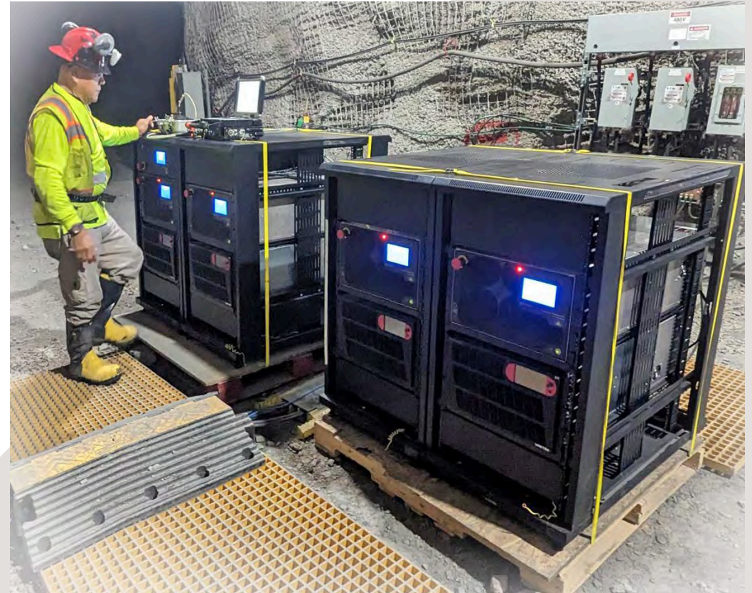
Four TerraTX-200 transmitters paired with 160 V / 188 A rectifiers, operating at 480 V.
