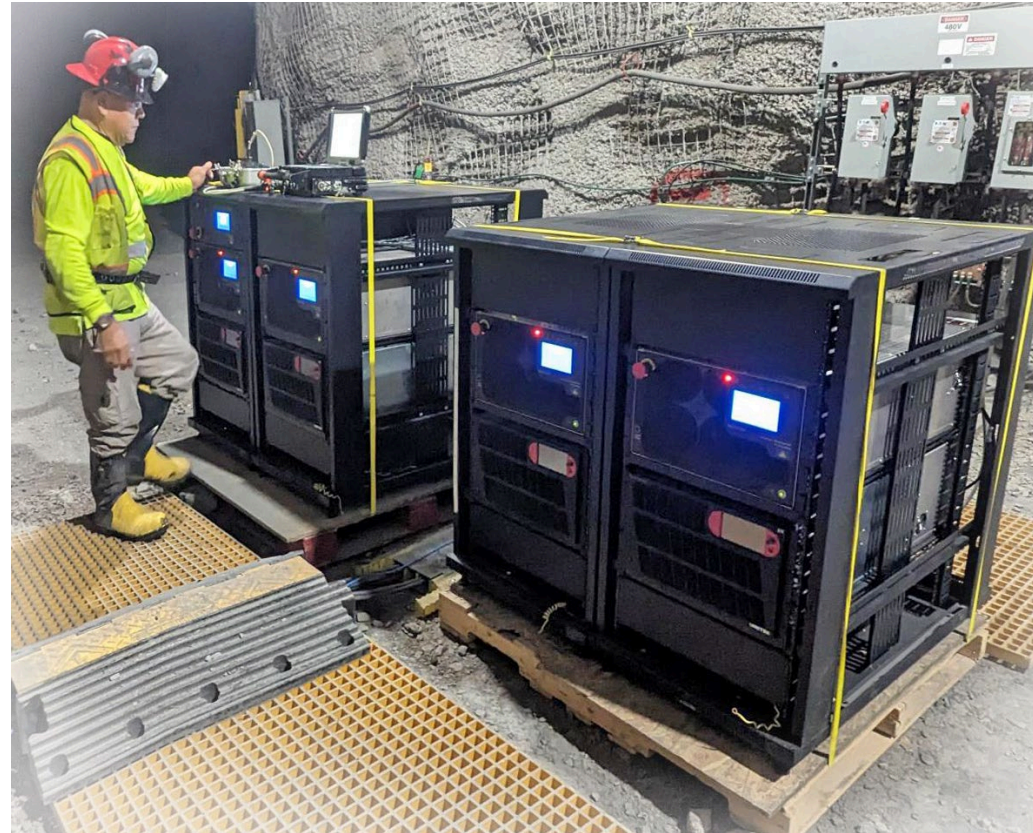
Four TerraTX-200 transmitters paired with 160 V / 188 A rectifiers, operating at 480 V.
